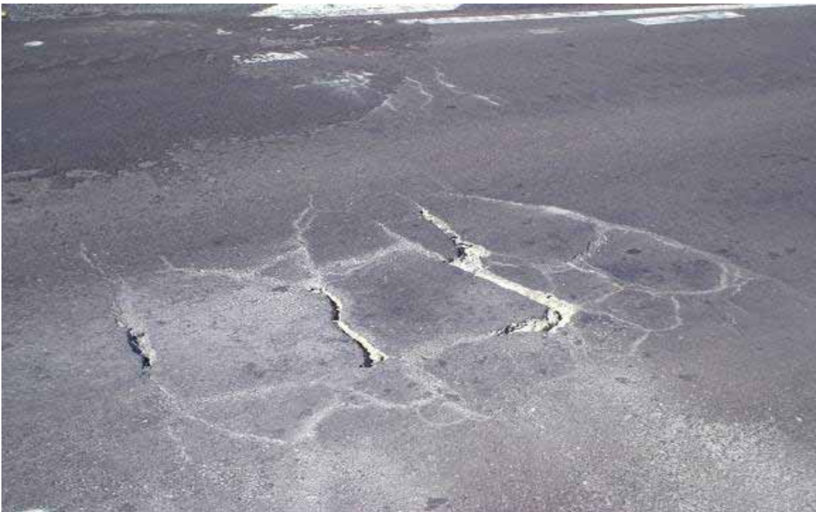
Figure 4.4: 18B Highway Patching & Cracking Issues
