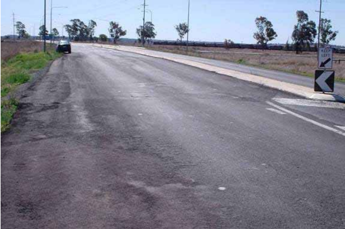
Figure 4.2: 18B Highway Roughness, Rutting & Shoving Issues
