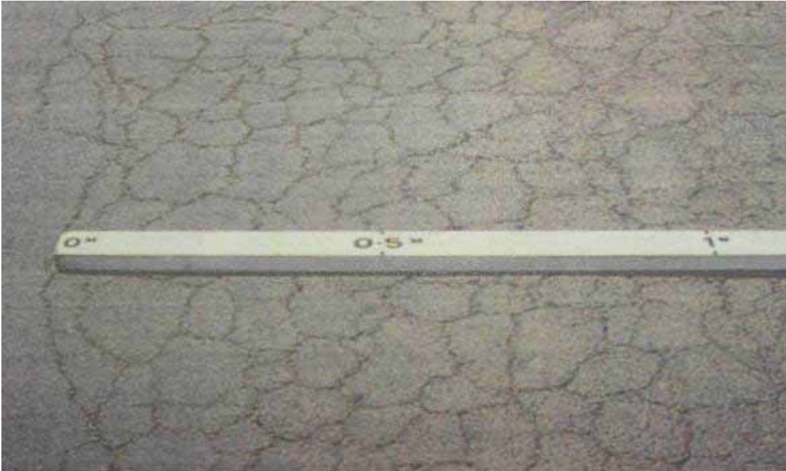
Figure 4.3: Crocodile cracking profile
