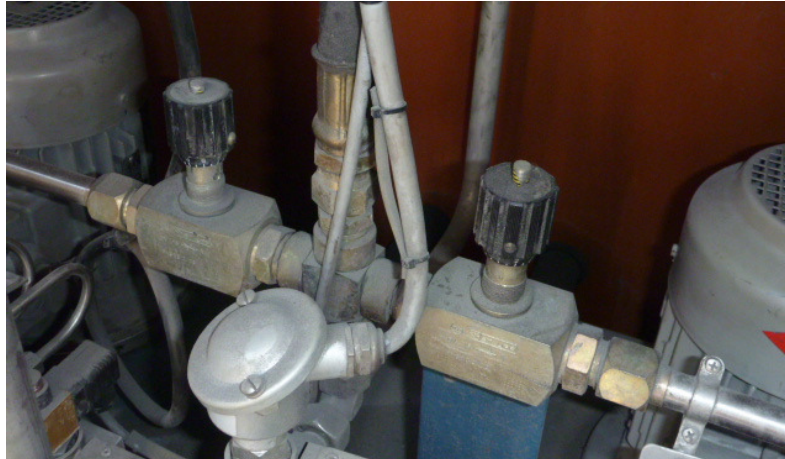
Figure 3.11: Two throttle valves located inside cabinet
