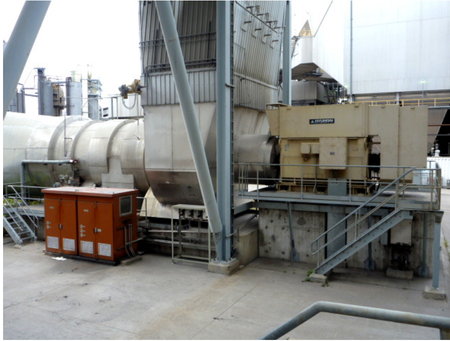
Figure 1.1: Callide C ID fan and induction motor
