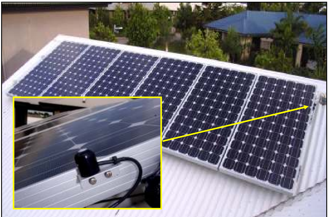
Figure 4.8 – PV Array and Pyranometer
