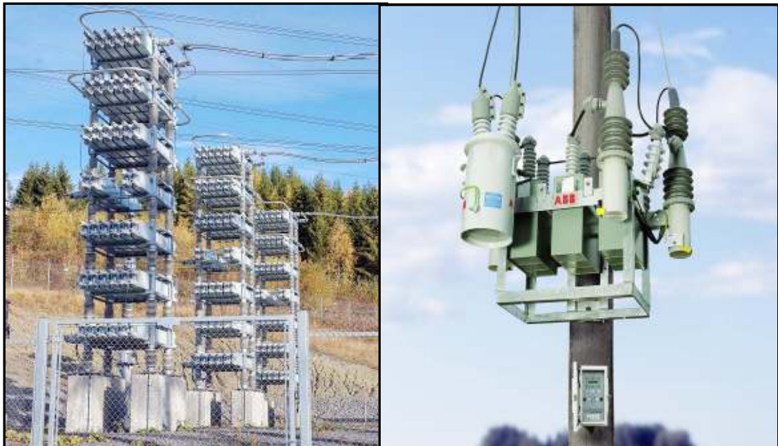
Figure 2.22 – Examples of Shunt Capacitor Banks (ABB 2010)
