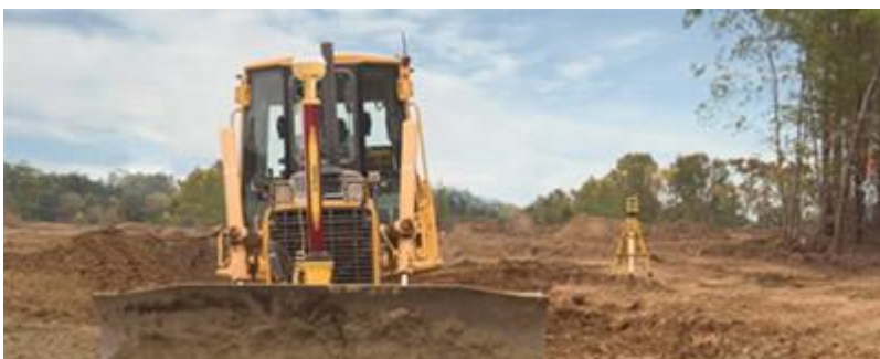
Figure 2.4: Trimble GCS900 on a Dozer with Single GPS and Laser Augmentation
