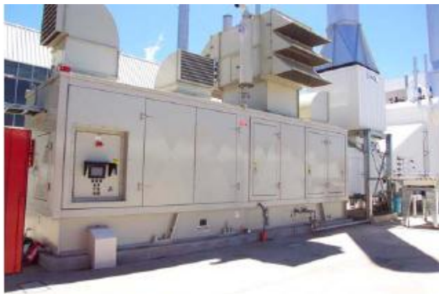
Figure 2.2: Natural gas turbine based co-generation plant by Sinklair Knight Merz [5] .
