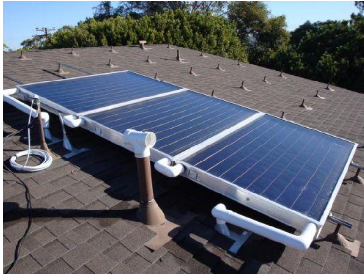
Figure 1.2 A sample FPC installation, (Source: HubPages 2010)
