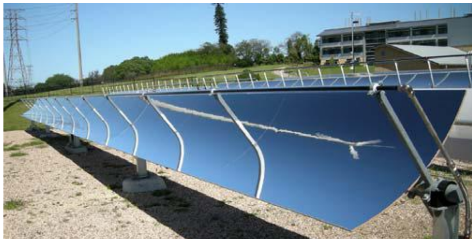
Figure 2.7 A sample PTC installation, (Source: NEP Solar)
