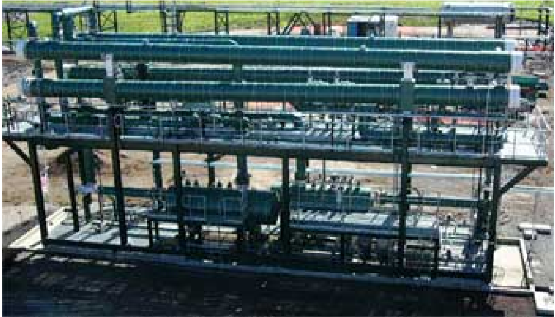
Figure 2.6: A dew point control unit installed at a gas processing facility. The JT valve is positioned at the bottom left of the photo. (adapted by Process Group, 2004)
