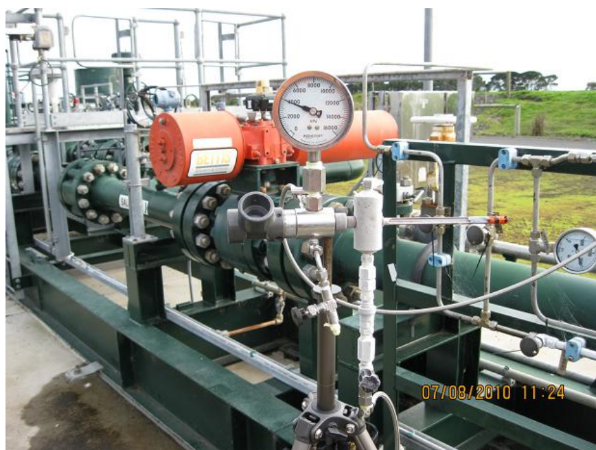
Figure 3.1: A Chandler MCFI in operation measuring the HCDP of an export natural gas. (Authors own photo)
