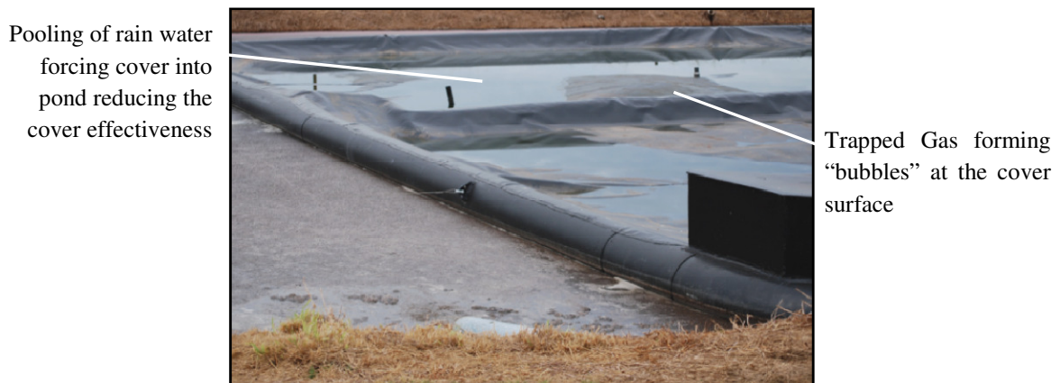
Figure 3-1 Existing pond cover with water and gas concentrations
