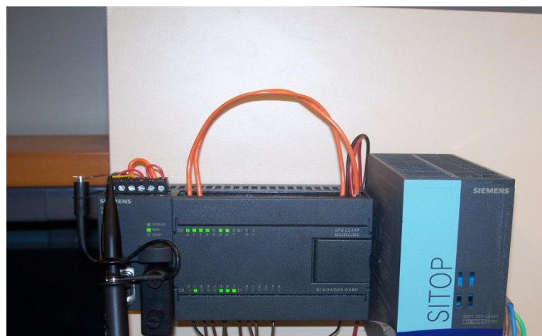
Figure 1.2: PLC in Operation
