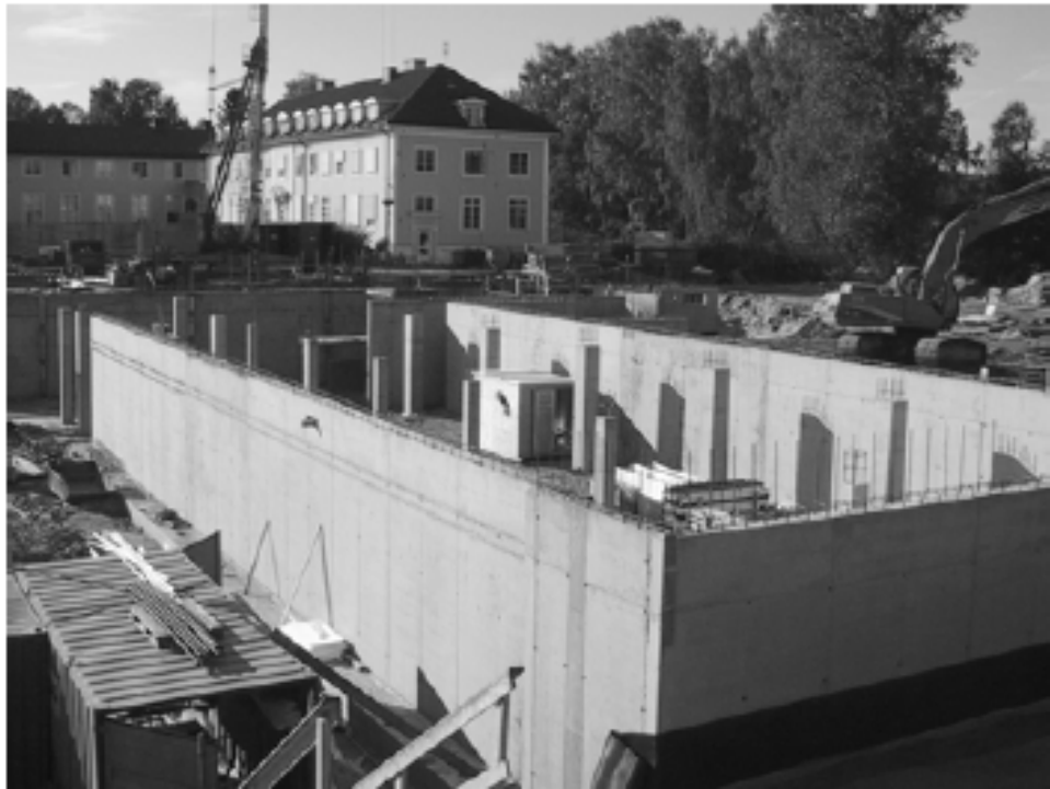
Figure 1.7: Construction of the New High School in Sorumsand, Oslo, Norway (Source: Mehus and Lillestol (n.d))
