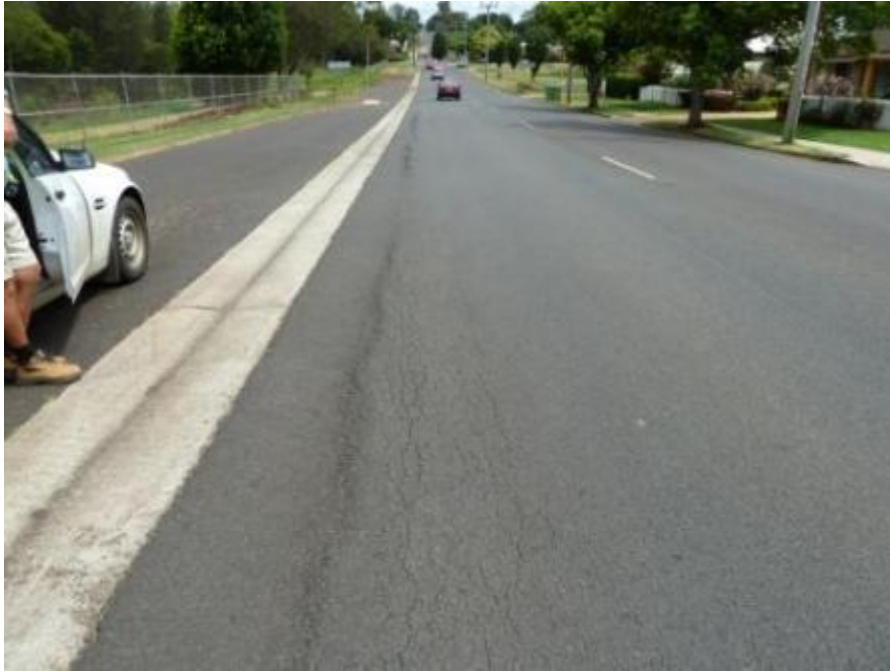
Figure 18 Mackenzie Street – rutting (Sourced: TRC NDRRA Photo file 2011)
