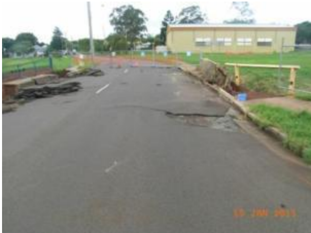
Figure 21 South Street - pavement lifting
