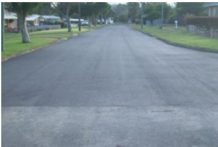
Figure 25 Teesdale Street - restoration works - 'mill and fill' (Sourced: TRC NDRRA Photo file 2011)
