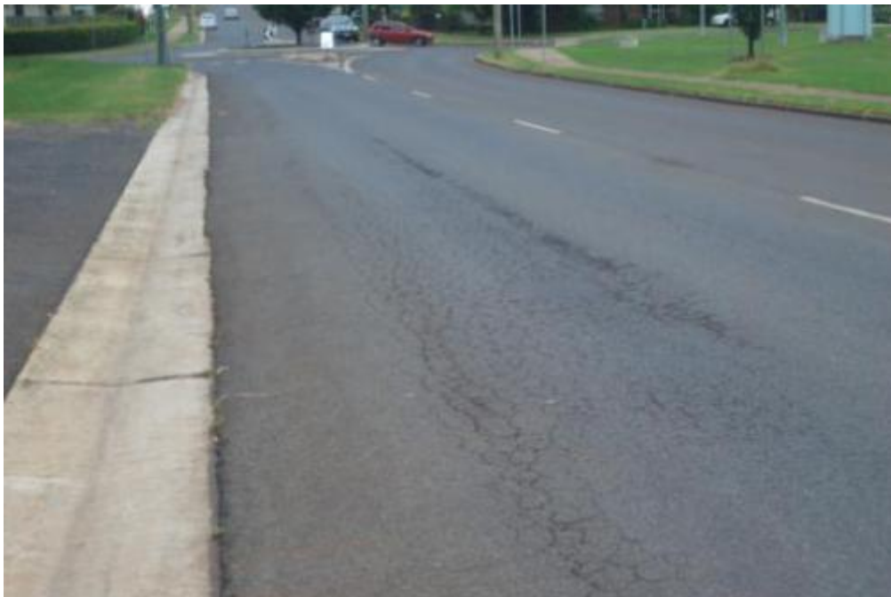
Figure 19 Mackenzie Street - crocodile cracking (Sourced: TRC NDRRA Photo file 2011)
