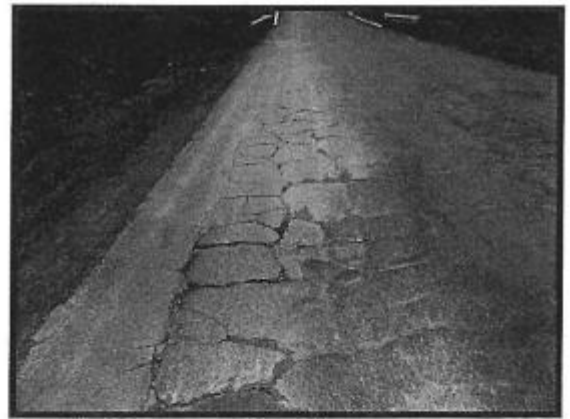
Figure 2 Pavement Crocodile Cracking
