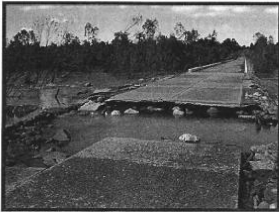
Figure 13 Damage to Floodway Structures
