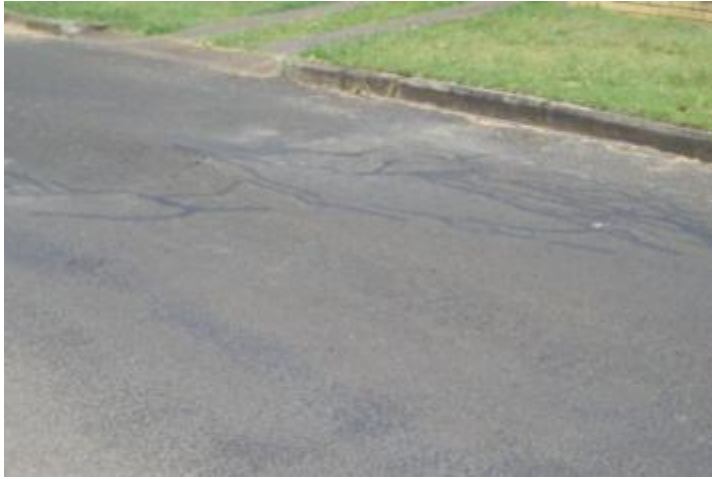
Figure 23 Teesdale Street - pavement flushing and stress cracking (Sourced: TRC NDRRA Photo file 2011)
