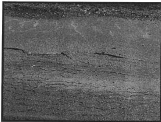
Figure 5 Pavement Stress Cracking
