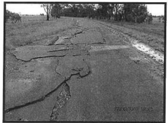
Figure 6 Lifting / Loss of Bitumen Seal
