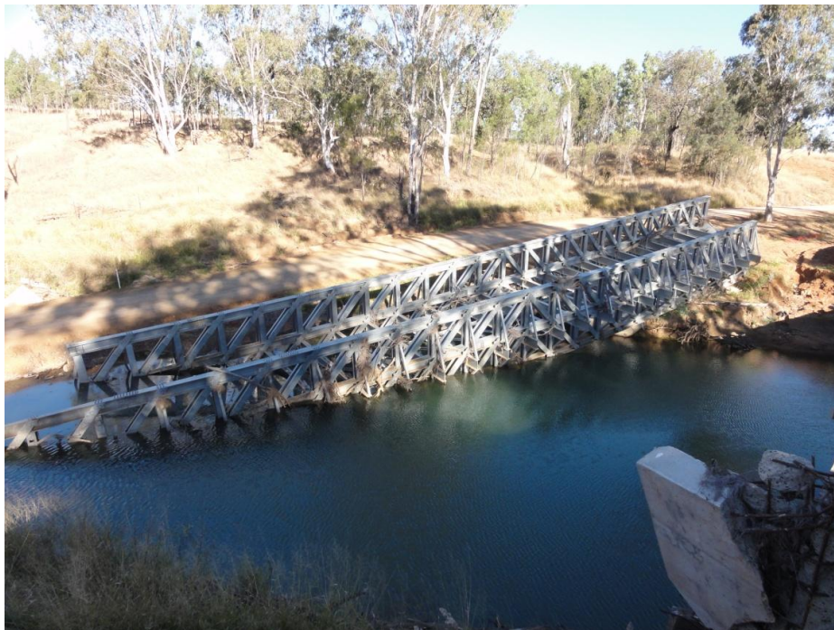
Figure 37: The existing steel truss bridge after being destroyed.
