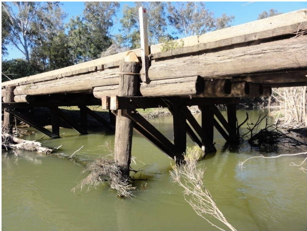
Figure 36: Jack Parr Bridge
