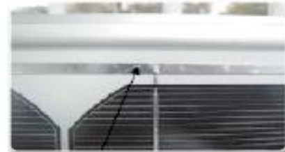
Note these Soldered joints have minimal coverage and barely cover the entire joint, this will create hot spots, potentially breaking the joint
