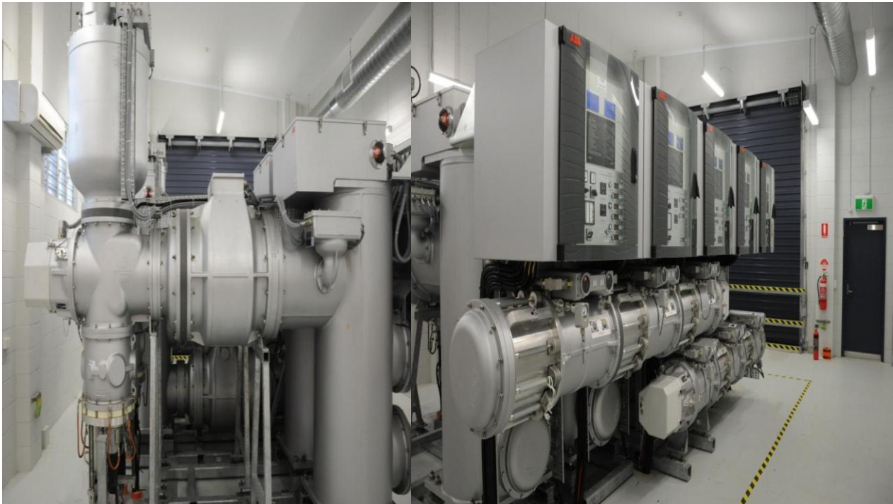
Figure 19: 66kV (GIS) Gas Insulated Switchgear (Ergon Energy, 2011)
