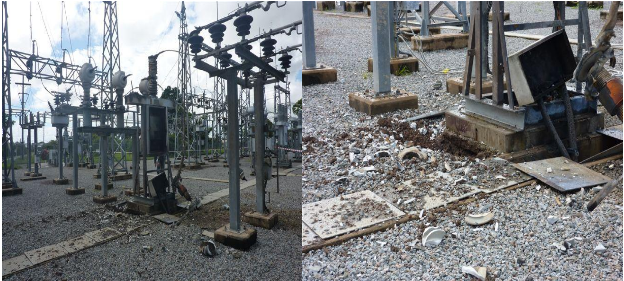
Figure 16: A typical substation clearance and equipment failure (Ergon Energy, 2011)
