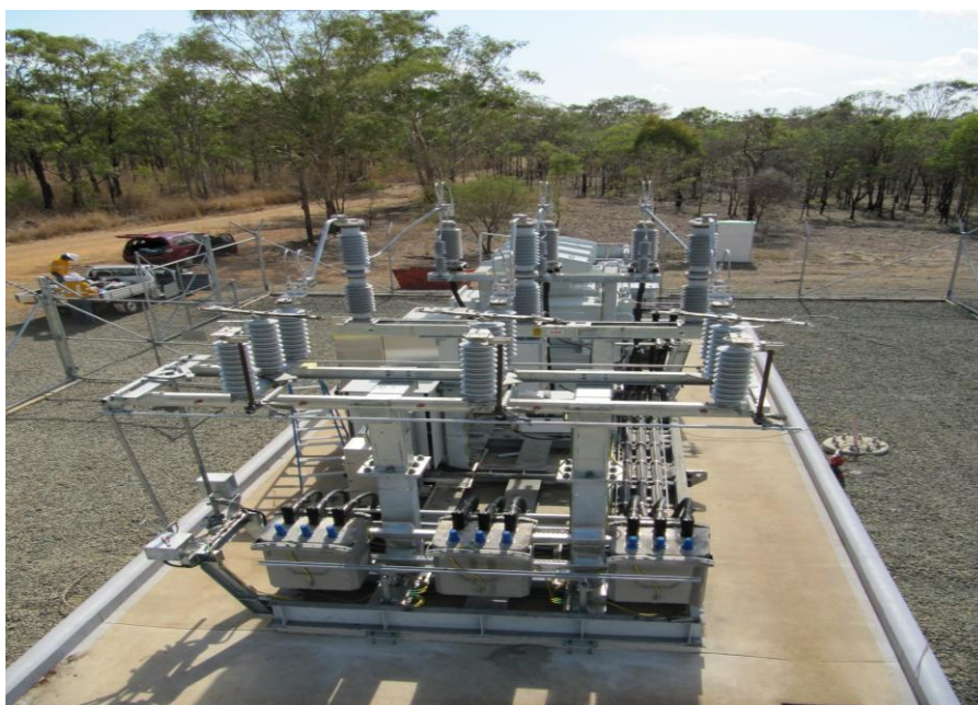
Figure 2: Skid Mounted Substation (Ergon Energy, 2011)
