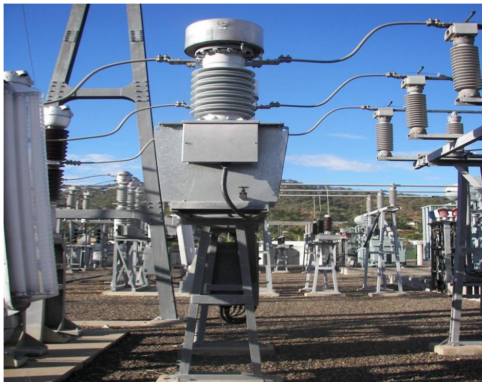
Figure 7: A typical outdoor HV Current Transformer (Ergon Energy, 2011)
