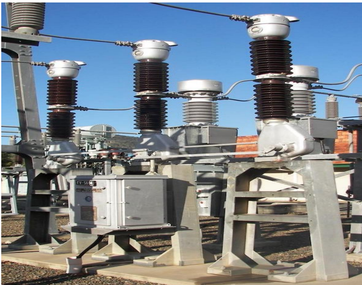
Figure 6: A typical outdoor 66kV “live head” circuit breaker (Ergon Energy, 2011)
