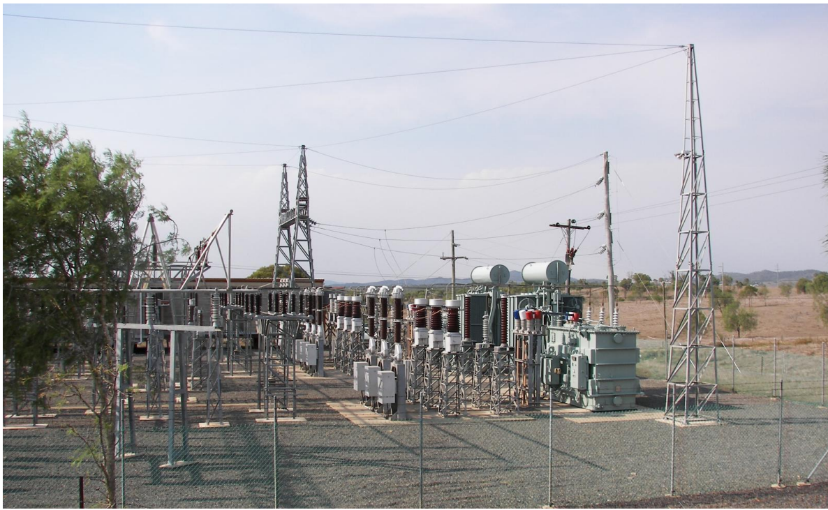
Figure 3: A typical 66/11kV zone substation (Ergon Energy, 2011)
