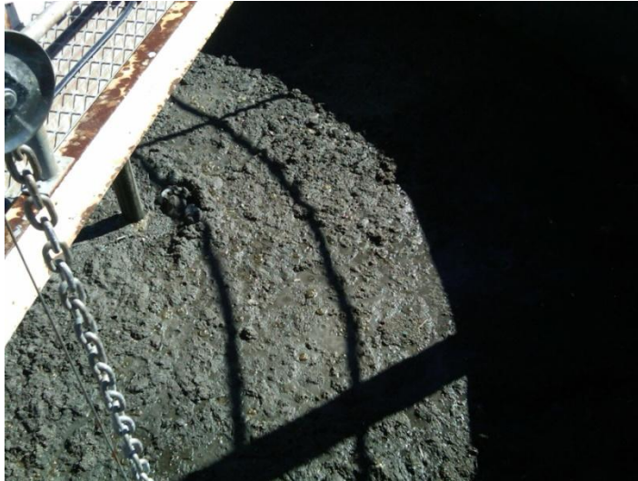
Figure 4.2: Scum layer with methane bubbles in anaerobic digester
