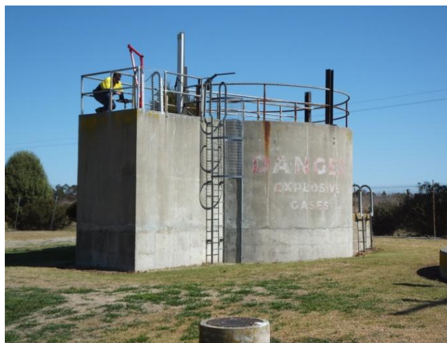
Figure 4.1: Anaerobic digester at Pittsworth Sewage Treatment Plant
