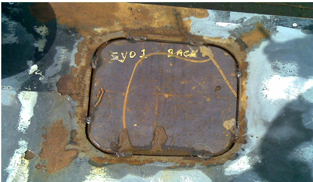
Figure 4-11 repaired section of pontoon where hold down bolts were pulled through
