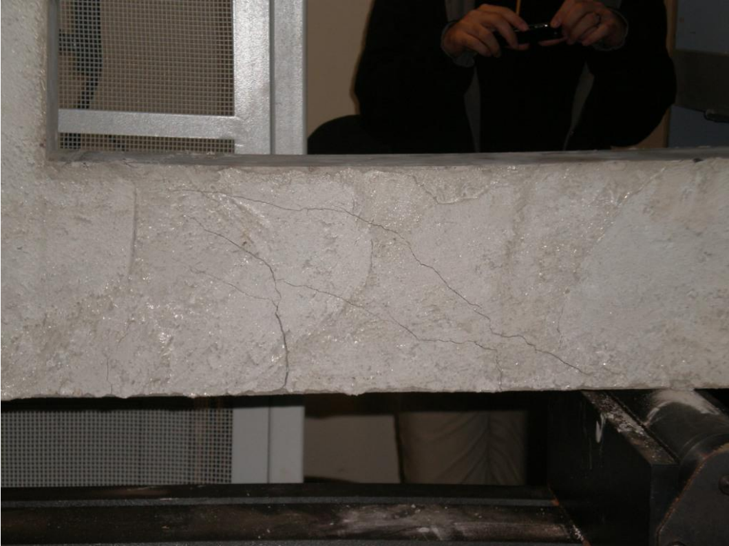
Photo 5 – Initial cracking in the optimum beam
