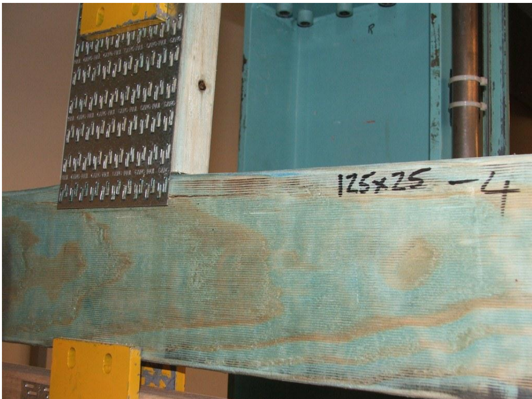
Figure 4.5 - ID1 with failure 100 mm either side of plate
