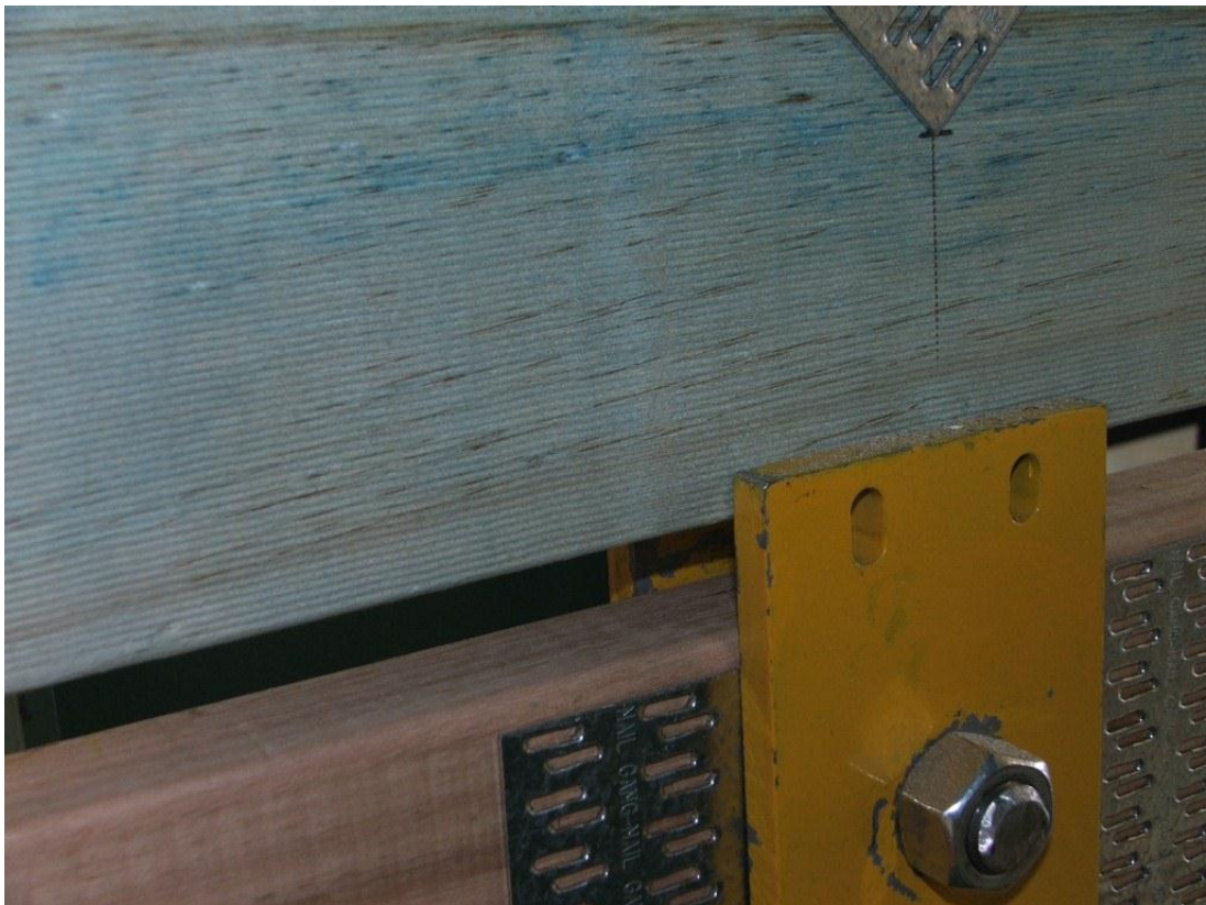
Figure 4.17 - Cracks appeared in area that was under compressive forces - bottom 1/4 of member
