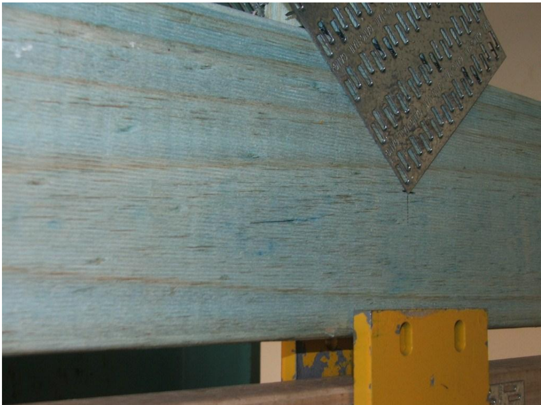
Figure 4.15 - Small crack appeared as dark lines at 8 - 10 kN
