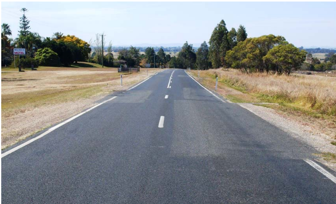
Figure 5.39 Gwydir Highway at Waterview showing patching
