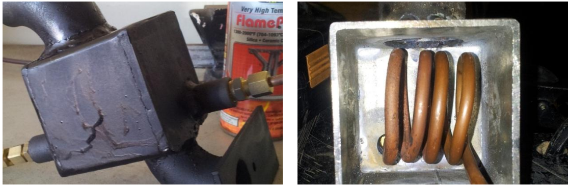
Figure 9: Exhaust water-to-steam heat exchanger on the left, and internal 6mm copper pipe coil inside the unit on the right.
