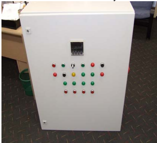
Outside of Control Panel
