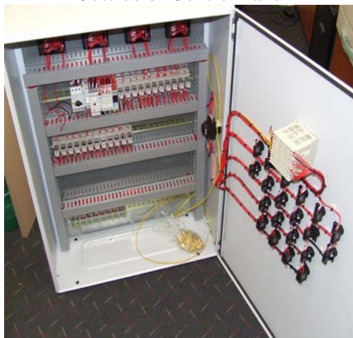
Inside of Control Panel
