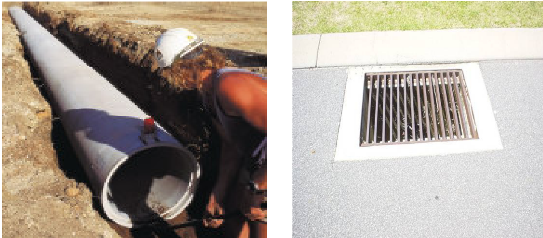
Figure 4-2 Typical Stormwater Drainage Infrastructure Assets
