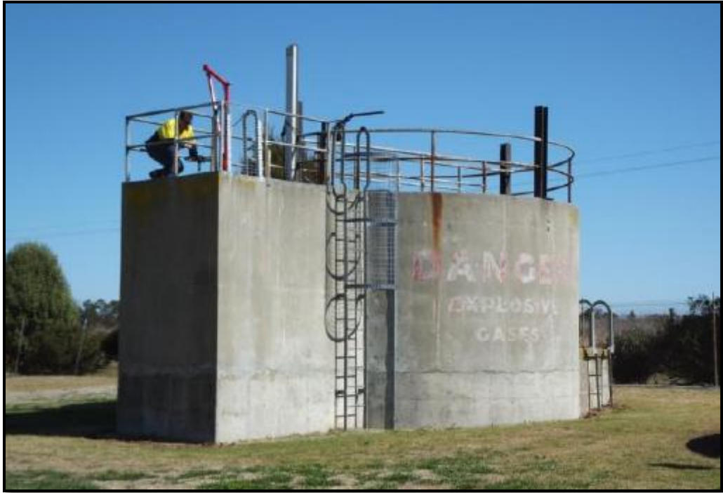
Figure 4 Anaerobic Digester Pittsworth
