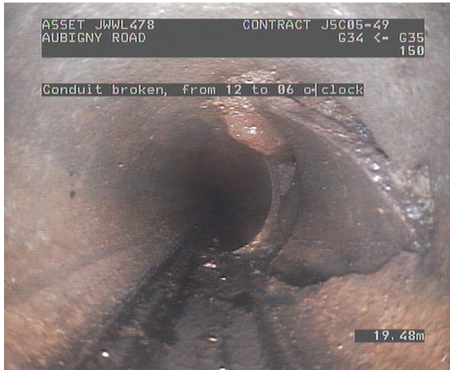
Figure 2-6 Image from camera work of the broken section of main
