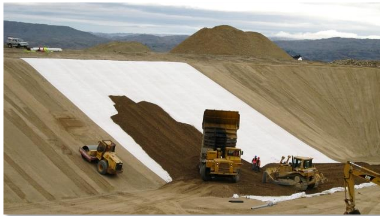
Figure 2.14: Geosynthetic Clay Liner (GCL) being installed on an embankment dam (source: www.geofabrics.com.au )
