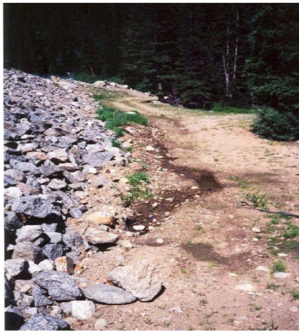
Figure 3.1: Seepage observed at Idaho Dam at downstream toe
