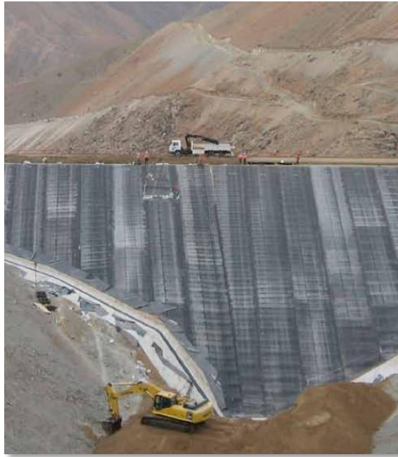
Figure 3.3: Bituminous geomembrane being installed on upstream face of embankment dam (source: www.coletanche.com )
