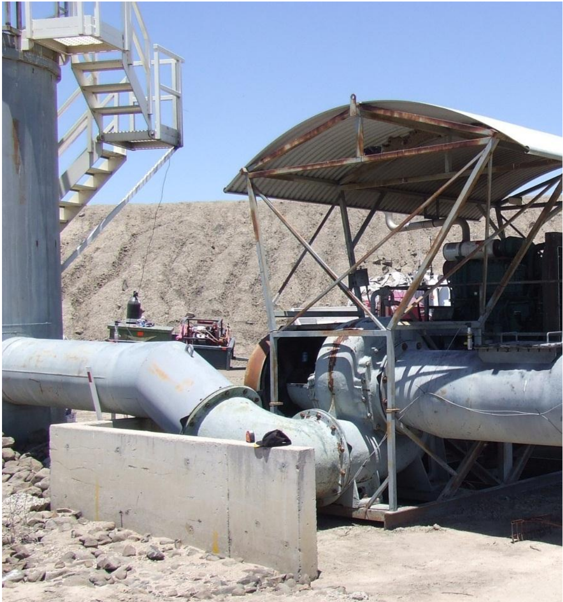
Figure 9: Pump station used for trial of pump efficiency monitor.
