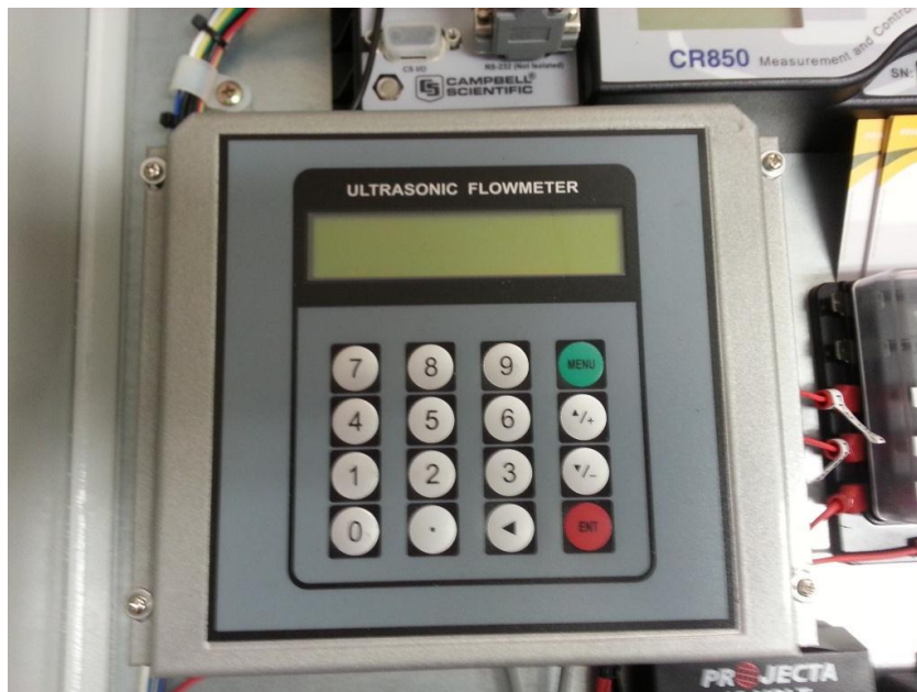
Figure 17: Display for ultrasonic flow meter.
