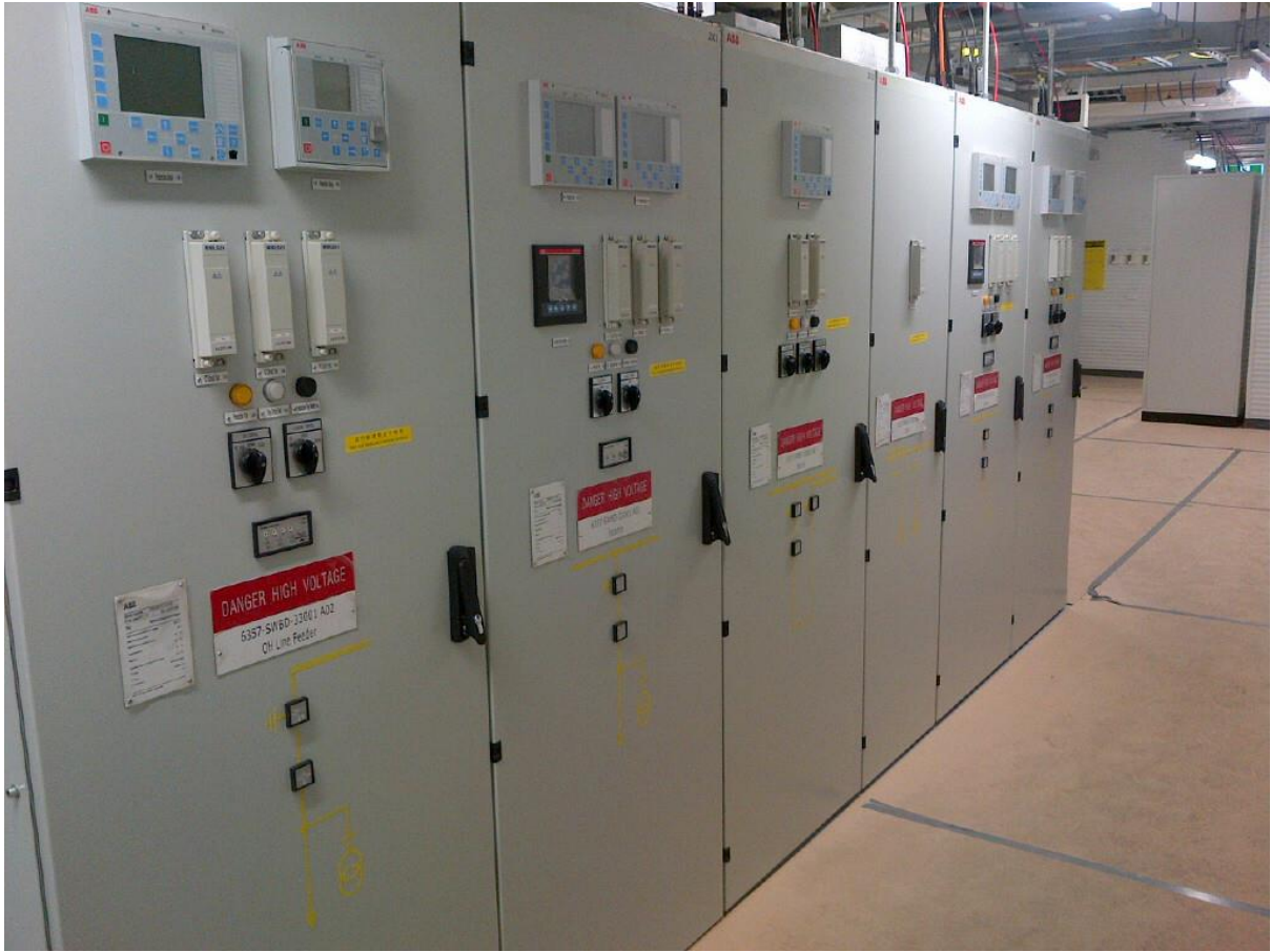
Figure 4.5 - 33kV Gas Insulated Switchgear (GIS) board
