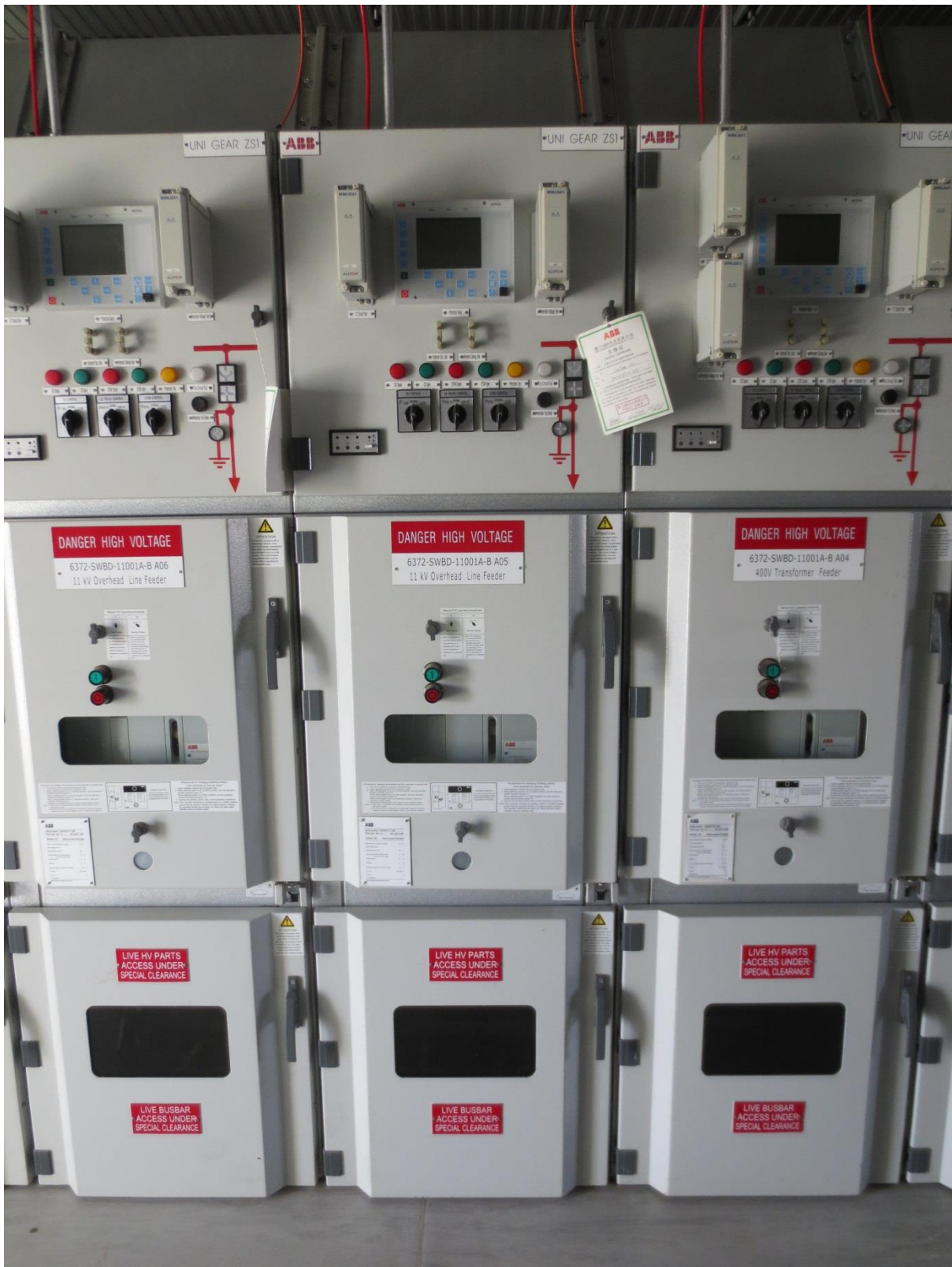
Figure 4.3 - 11kV Vacuum Circuit Breaker (VCB) board
