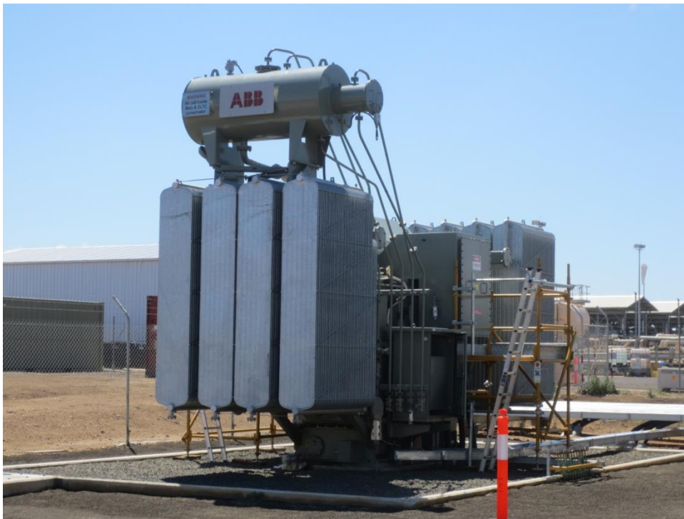
Figure 4.1 - 11kV/33kV 16MVA YNd1 transformer
