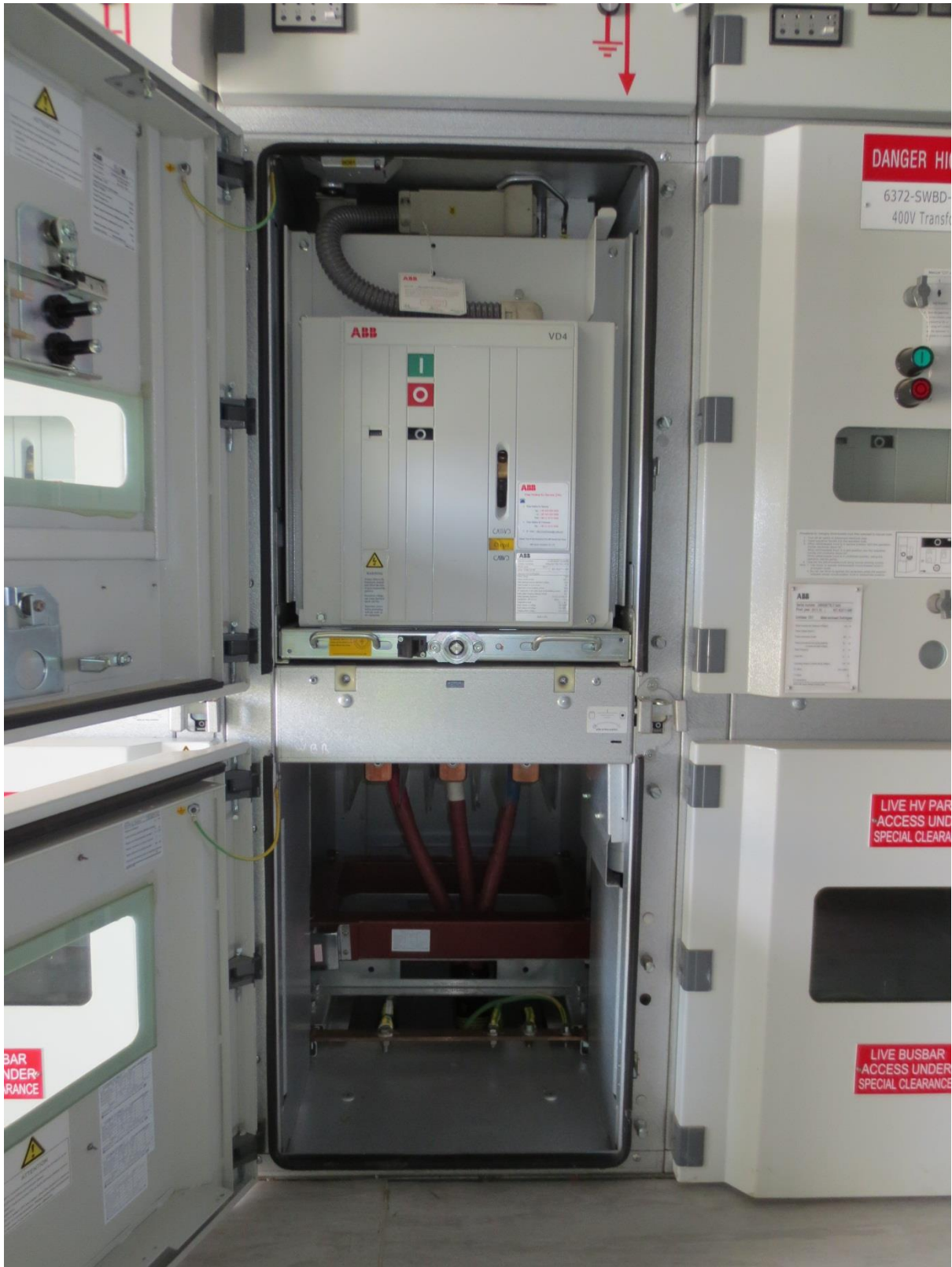
Figure 4.4 - 11kV Vacuum Circuit Breaker (VCB) showing internal arrangement, including cable connection
