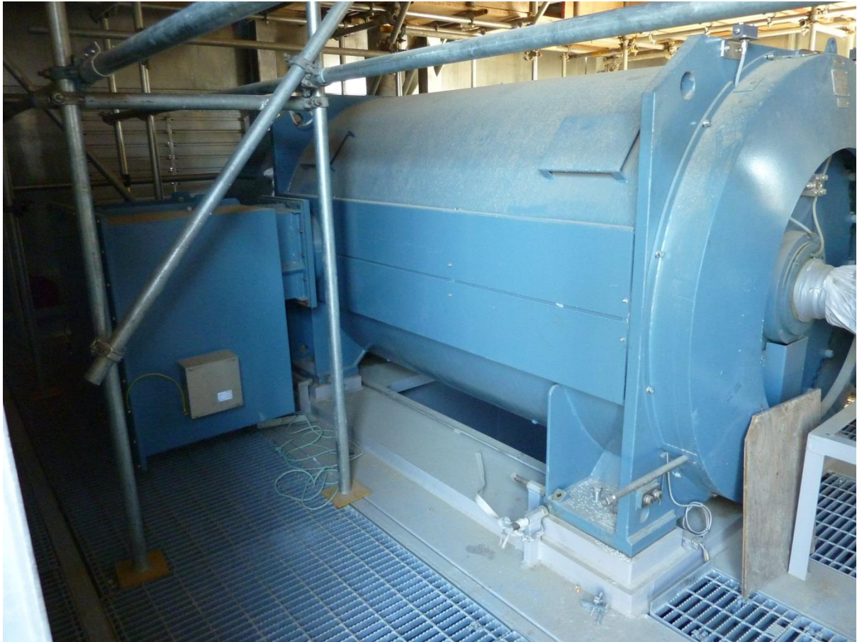
Figure 4.7 - 11kV 2.675MVA electric motor
