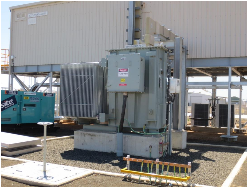
Figure 4.2 - 11kV/415V 2.5MVA Dyn11 transformer
