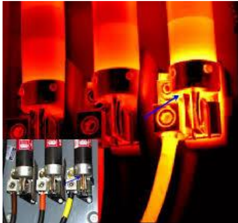
Figure 2.2 – Thermographic image of fuse cartridge assembly
