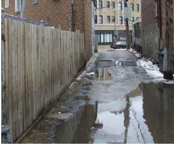
Figure 4.8 - A Chicago alley before conversion into a 'Green Alley' (Chicago Department of Transportation 2010).
