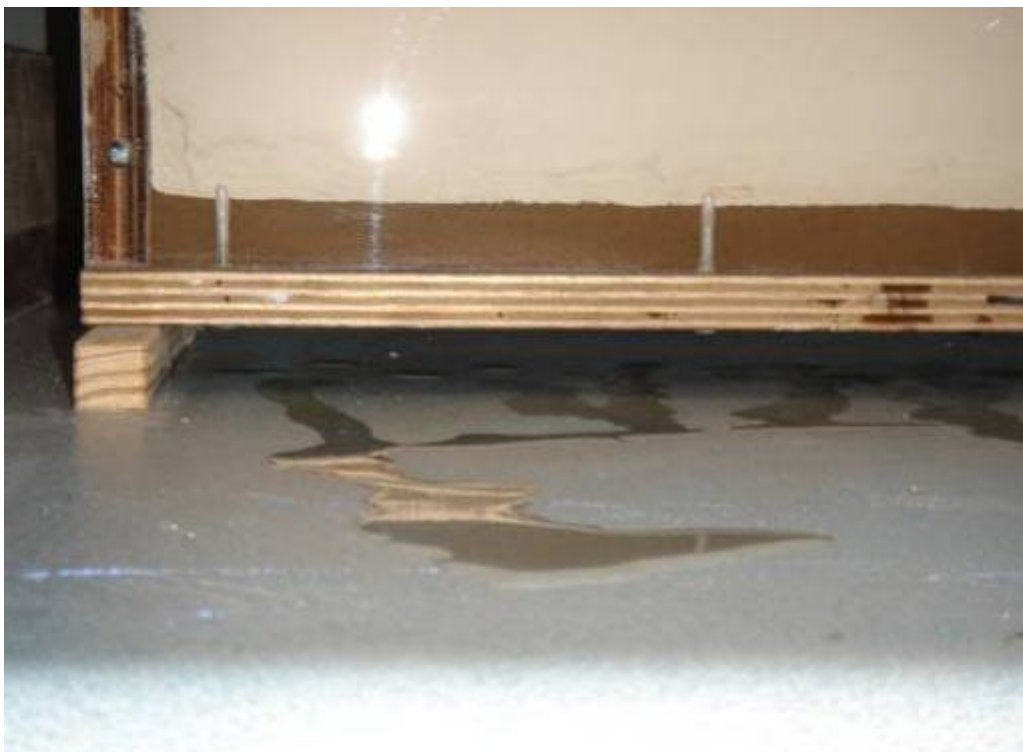
Figure 2.32: Water dripping from the bottom drainage holes.
