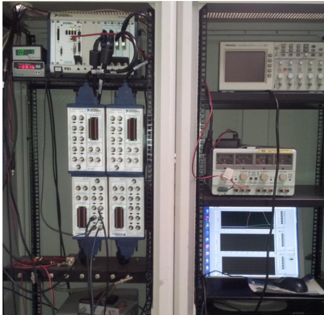
Figure 4.10: Overall view of the data acquisition system
