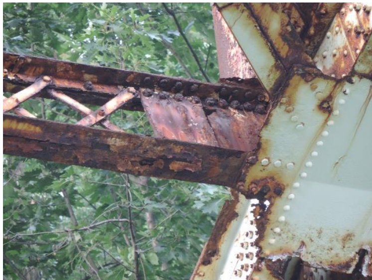
Figure 2 – Deteriorated steel (A. Davies, 2003)
