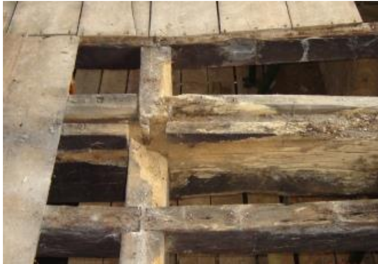
Figure 3 – Deteriorated wood/timber (J. Hoath, 2006)
