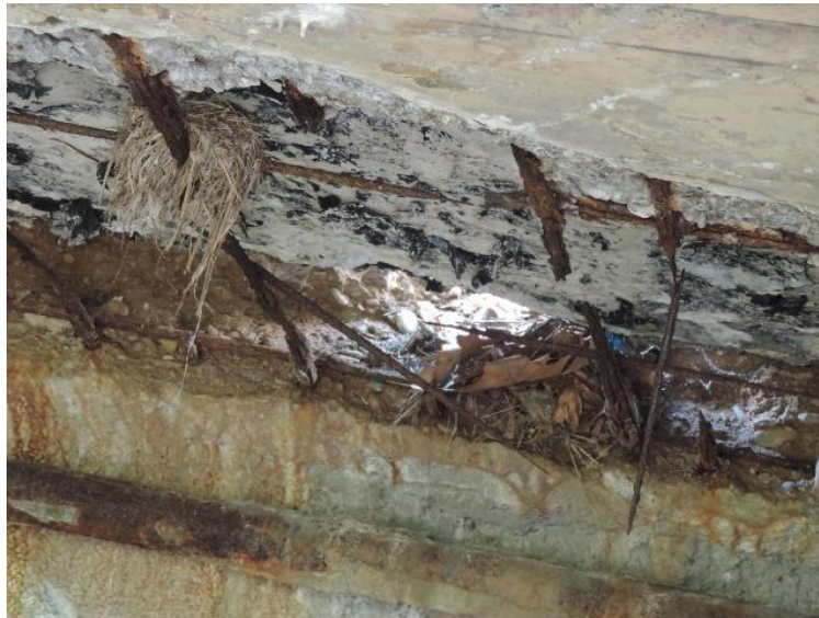
Figure 1 – Deteriorated concrete (A. Davies, 2003)
