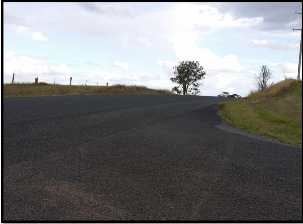
Figure 5- 13: Entering a 100 km/hr road with only an 80 metre sight distance. Anthony Road/Roadvale-Harrisville Road intersection.
