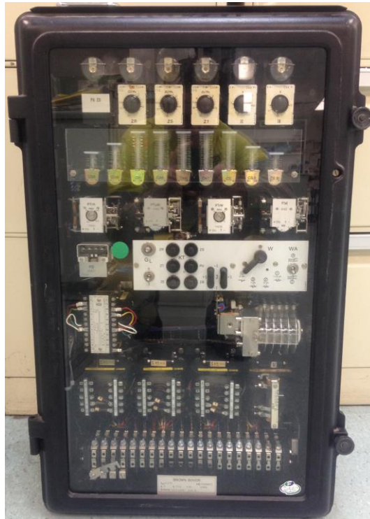
Figure 1: Electromechanical Distance Relay (Brown Boveri LZ32)
