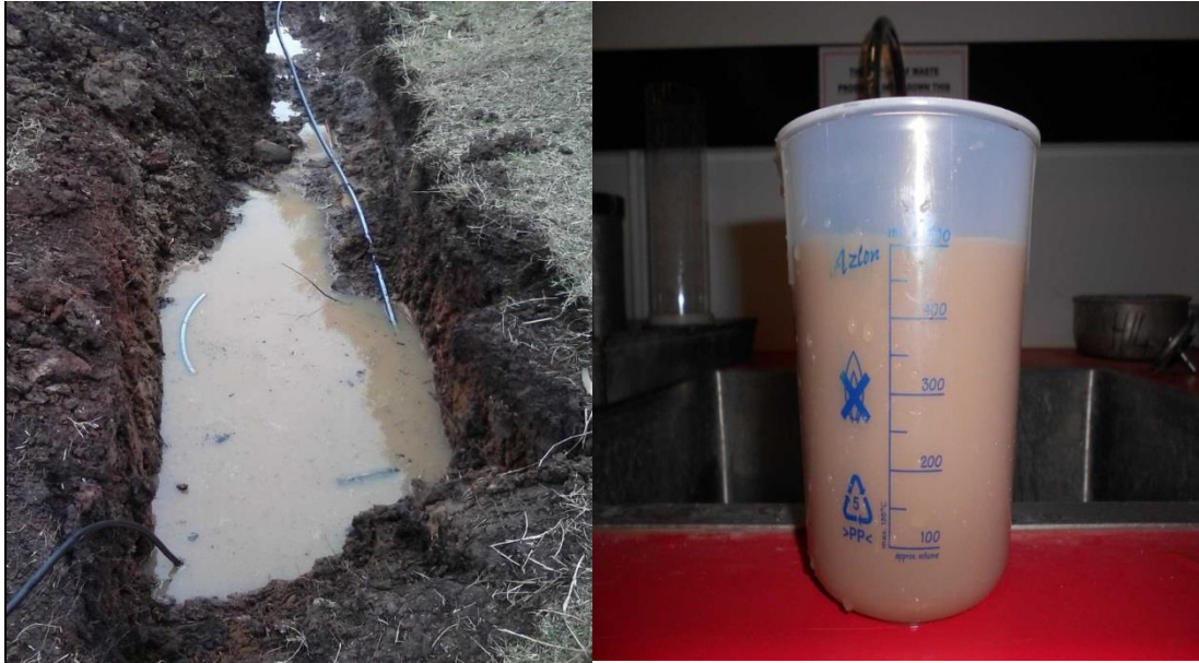
Figure 13: Pictures depicting the contamination of water used for FHT. Clay content was as a consequence of erosion resulting in high turbidity levels.
