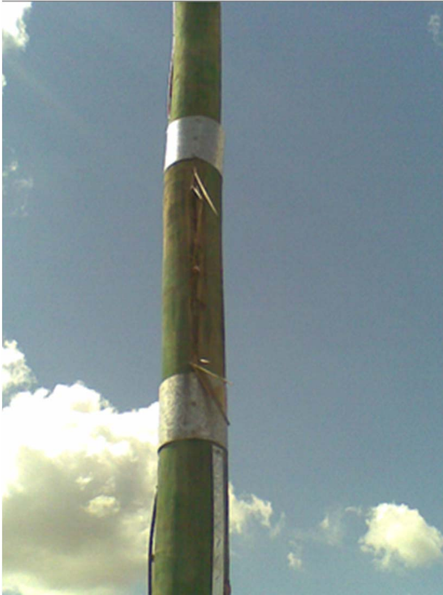
Figure 3.2 - Example of splintering between the Gapped Bands
