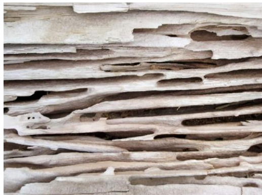
Figure 7: Termite affected wood
