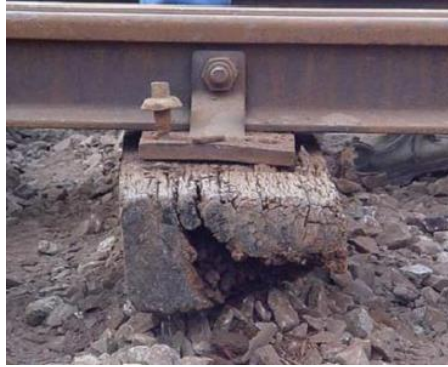
Figure 5: Failure due to fungal attack (Ferdous & Manalo 2014)
