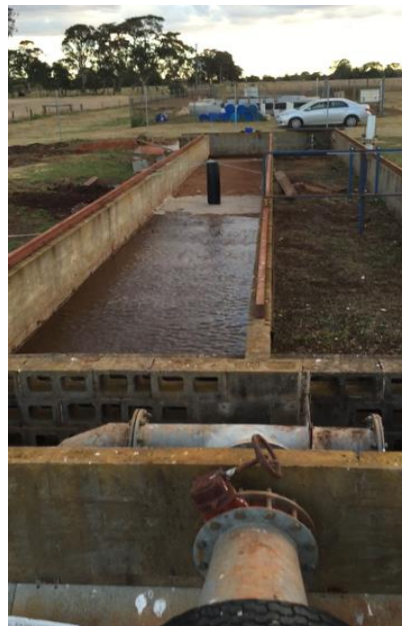
Figure 4.14 Flume Control Valve slowly opening showing water flow
