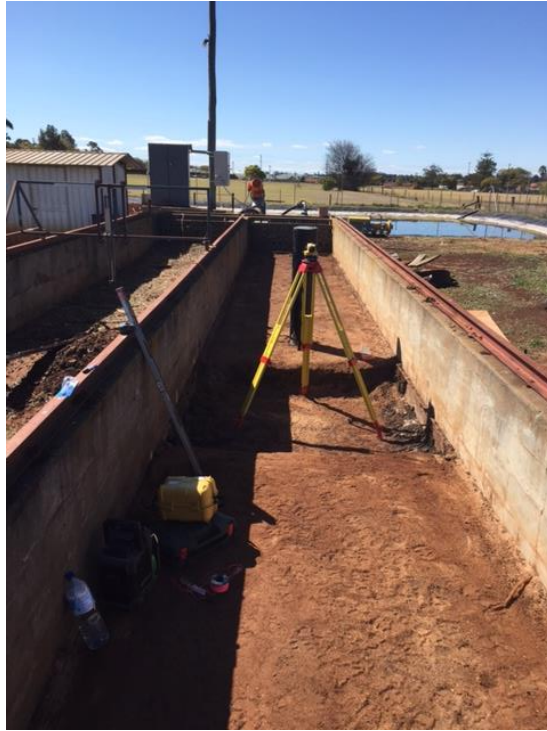
Figure 4.12 Excavation of Flume showing area of interest dug at 0.300m below flume bedding level
