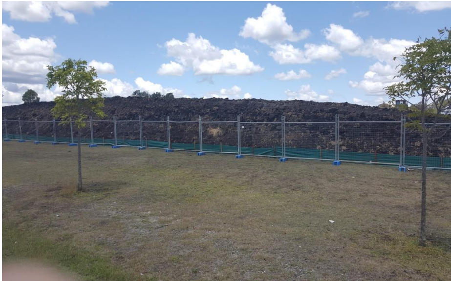
Figure 13: Geotextile sediment fence
