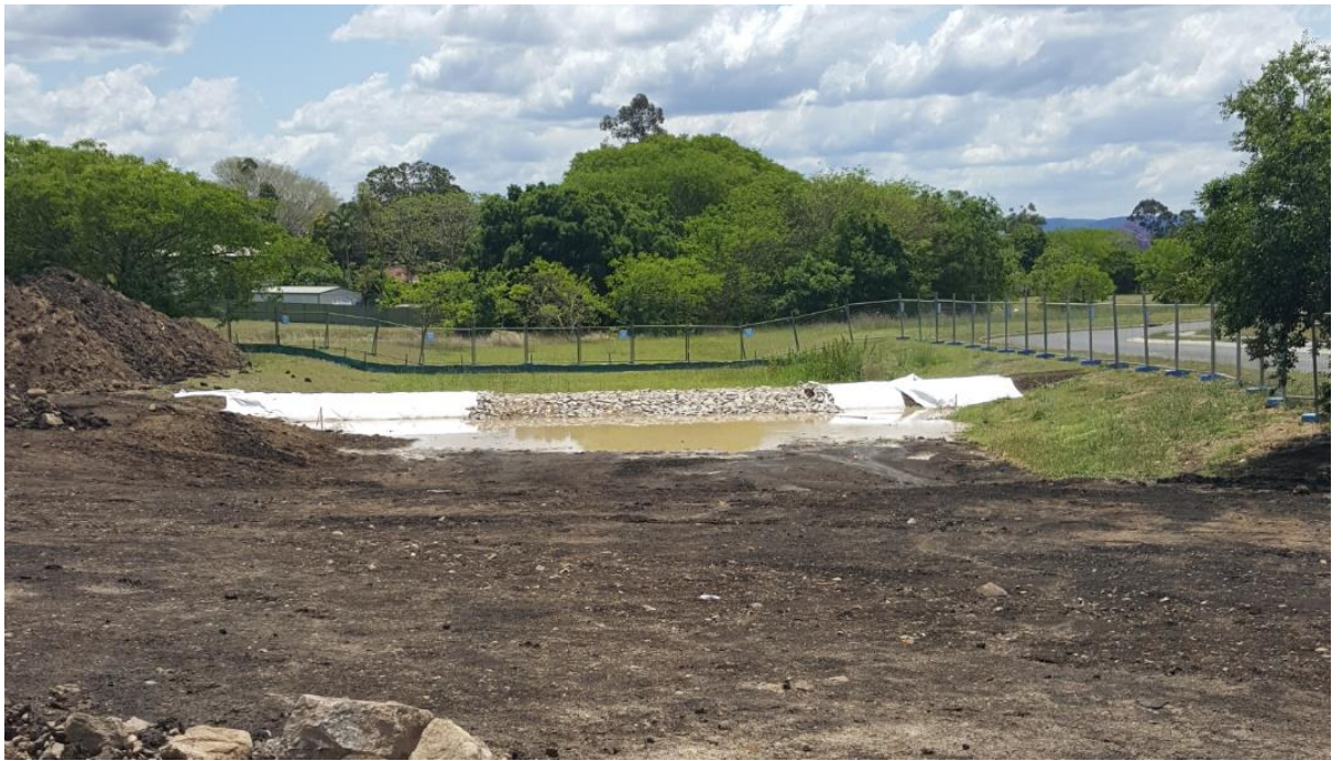
Figure 14: Sediment control wall
