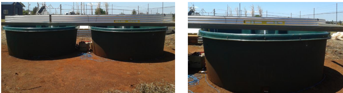
Figure 3.9: Tanks were levelled using a split-level and a section on steel tube placed across the top edge of the two tanks
