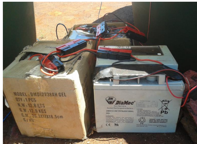
Figure 3.3: 12 volt battery supply
