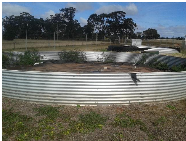
Significant vegetation and weed growth occurred around tank perimeter
