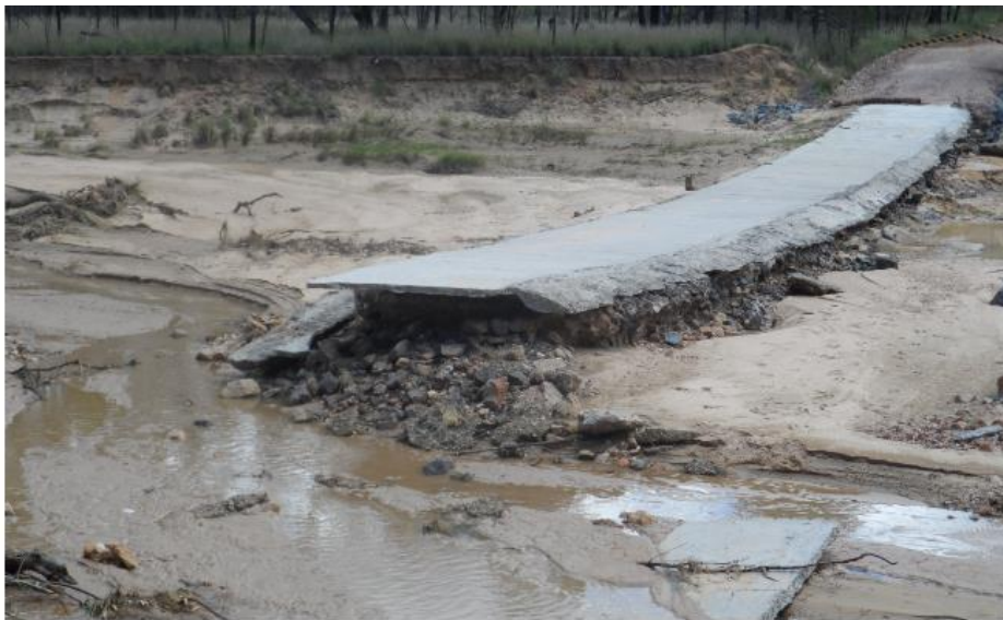
Figure 2.17: Floodway Damage (Scour) (Queensland Reconstruction Authority n.d.)
