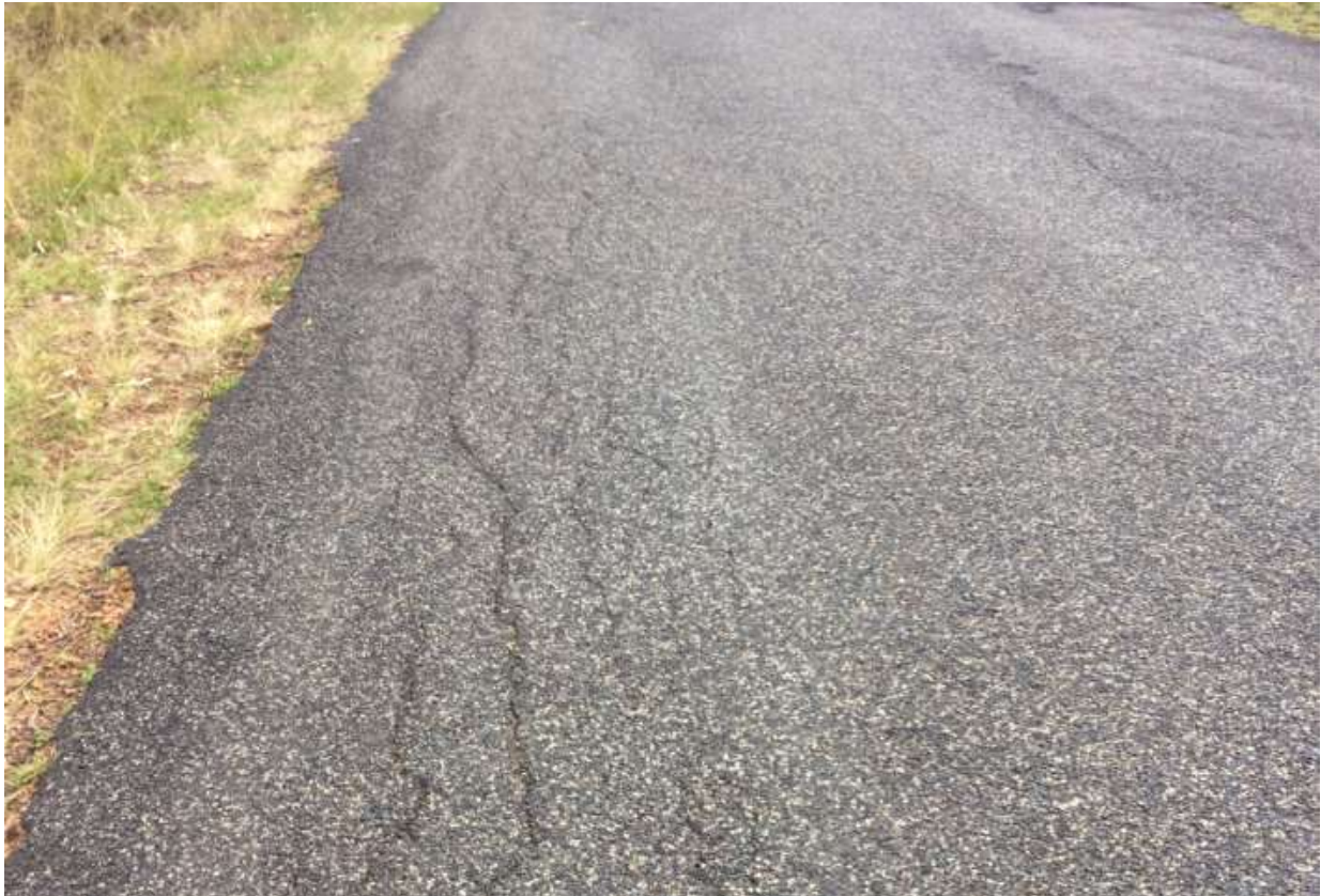
Figure 2.11: Example of distress cracking on local road.
