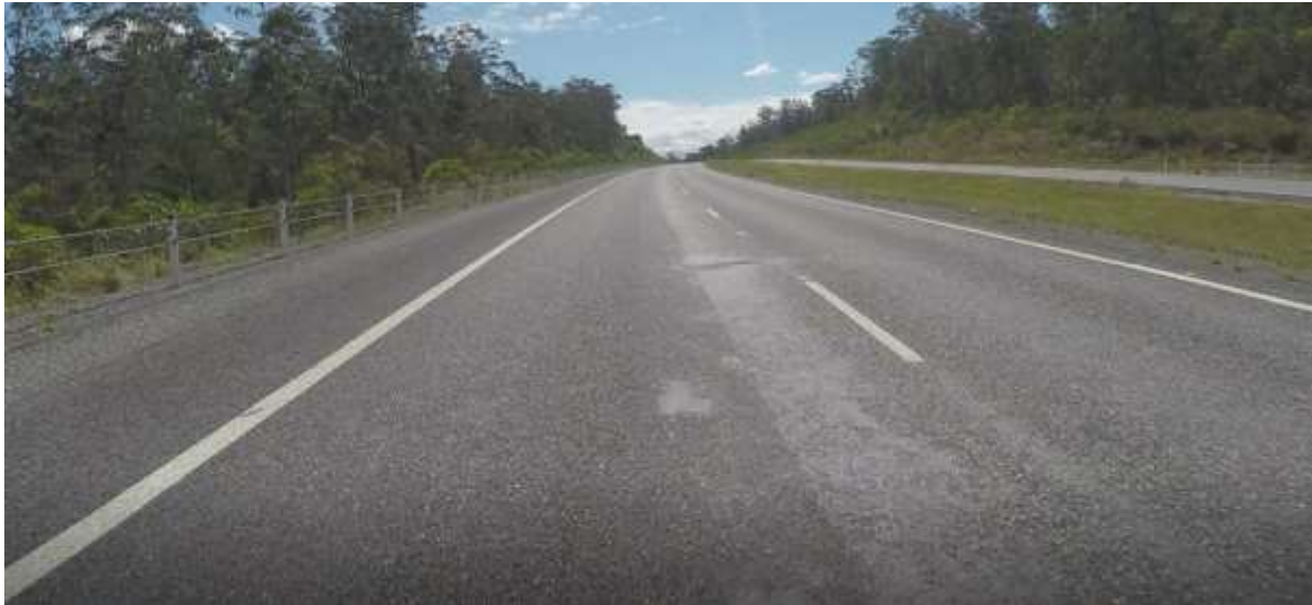
Figure 4.4: Image from the video used for the defect mapping, heavy patch can be seen of the left side of the image.
