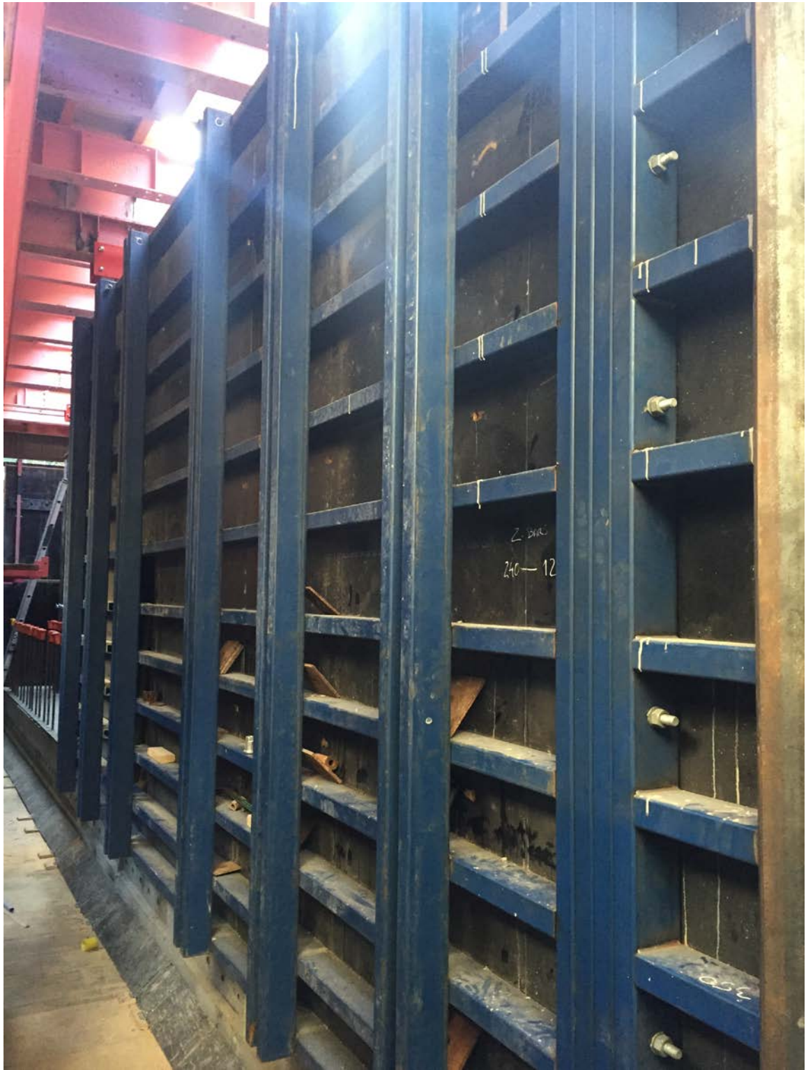
Figure 2-12 Steel Frame RHS wall forms within jump form at 300 George St Brisbane
