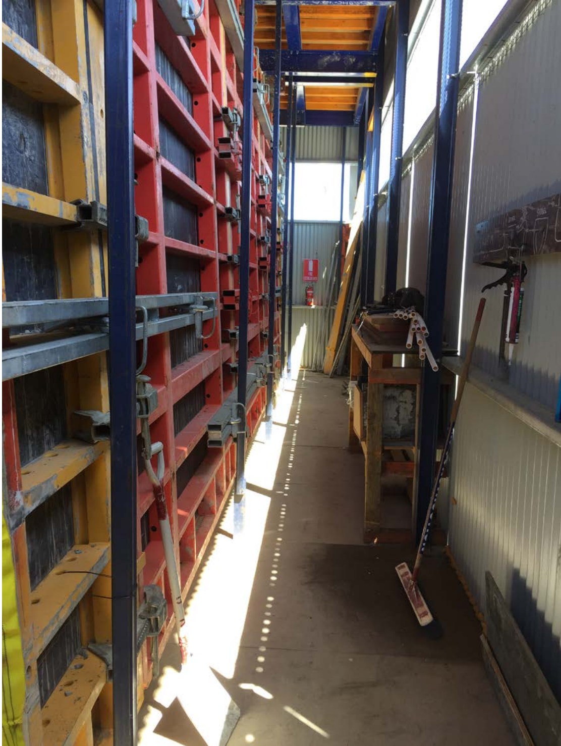
Figure 3-5 Peri Modular Panel Forms within Jump Form at Crown Towers Project Perth WA
