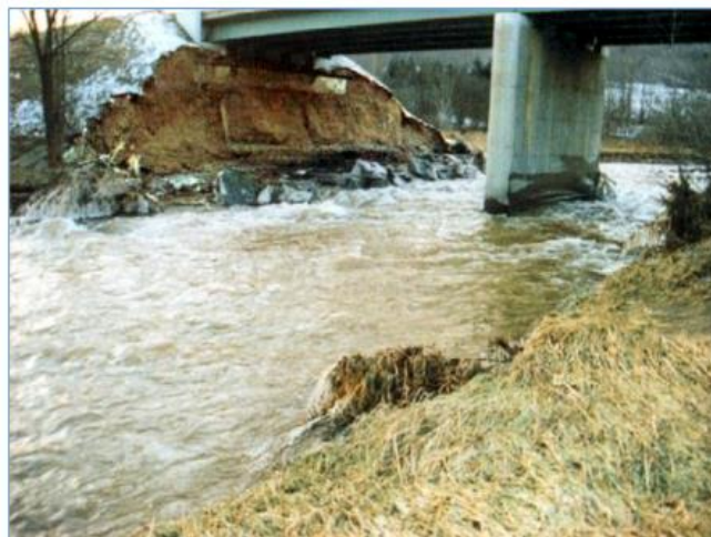
Figure 3.9, Geotechnical failure of spill-through abutments (Ettema et al. 2006)
