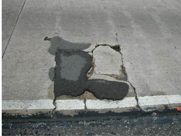
Figure 2: Example of pavement punch out and an attempt to patch.
