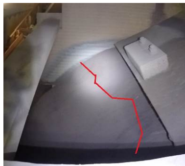
(b ii) Fracture line
