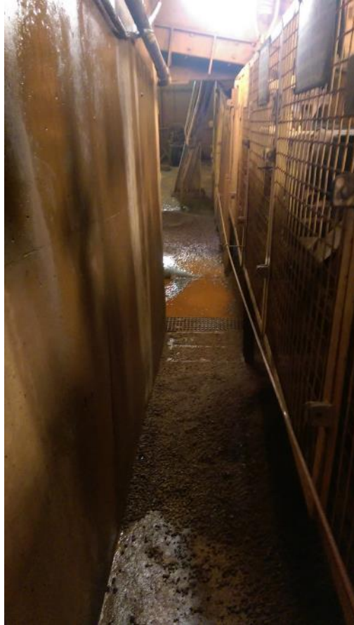
Figure B-1 Spillage adjacent to chute outlet.
