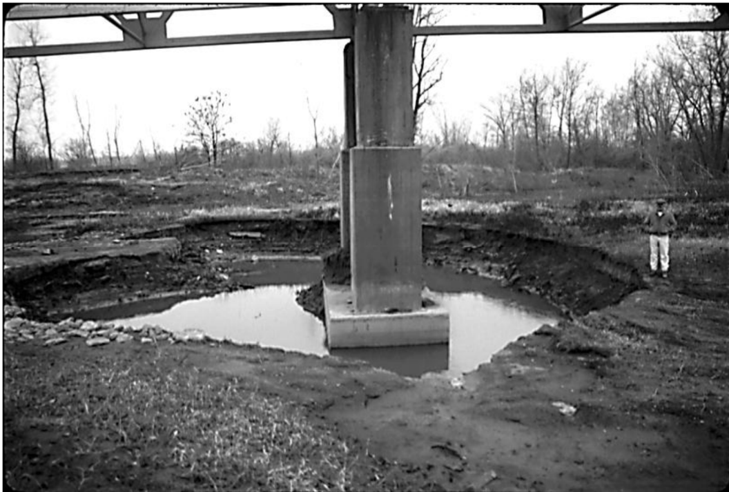
Figure 1.1 Local scour around a bridge pier (FDOT 2005).
