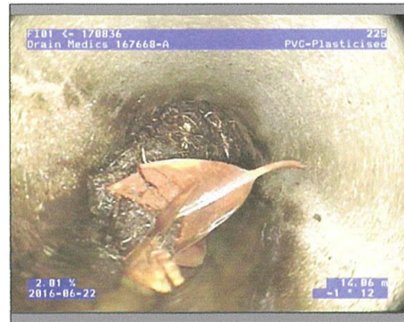
Photo: 1_10A 14.06m, A Mass of mostly fine Roots, which has developed into an interwoven clump, at joint, Obstruction: 51-75% , from 6 to 3 o'clock
