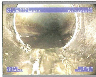
Photo: 1_4A 0.8m, Recently Cut interwoven mass of mostly fine roots leaving a Beard of roots, at joint, Obstruction: 5-20% , from 4 to 8 o'clock
