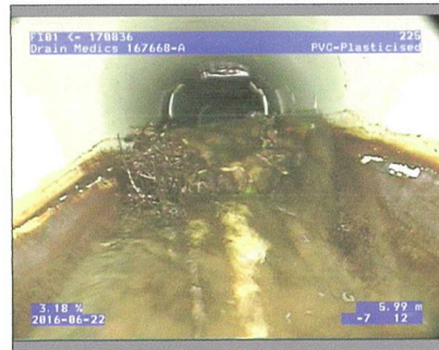
Photo: 1_5A 5.99m, Recently Cut interwoven mass of mostly fine roots leaving a Beard of roots , Obstruction: 21-50% , from 4 to 8 o'clock
