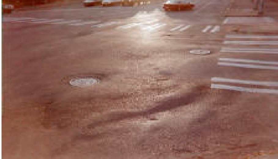
Figure 4.2.2. Road Pavement Shoving
