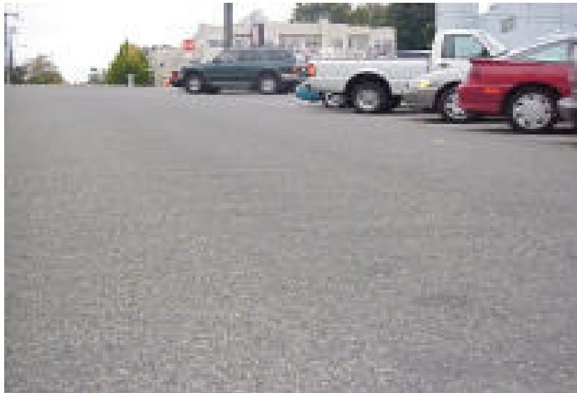
Figure 4.2.3. Road Pavement Corrugations
