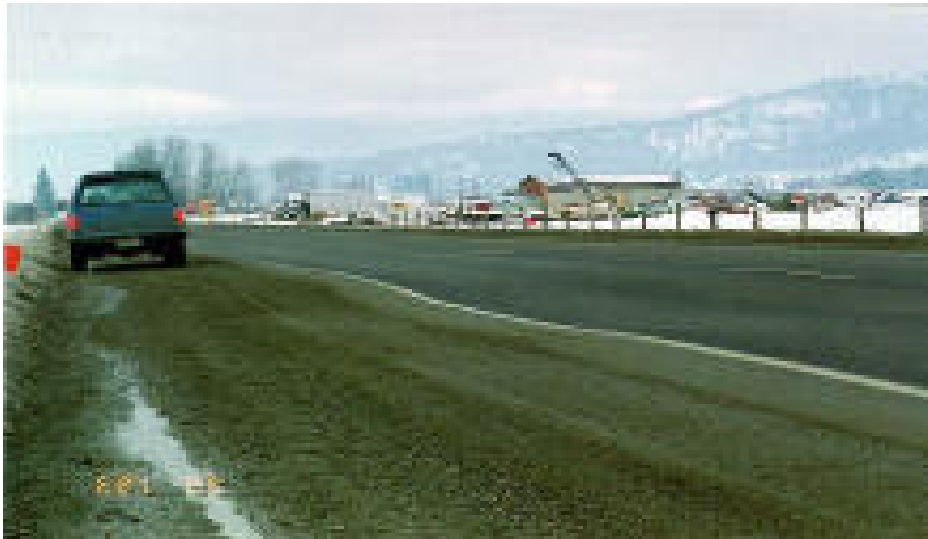
Figure 4.2.0 Road Pavement Depression
