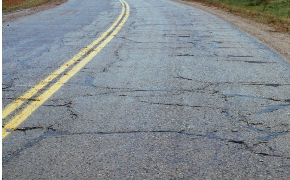
Figure 4.2.4. Block Cracking SOURCE hotmix.ce.washington.edu
