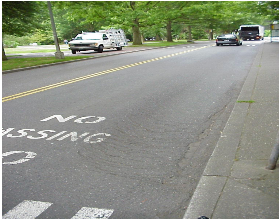
Figure 4.2.6 Crescent Shaped Cracks
