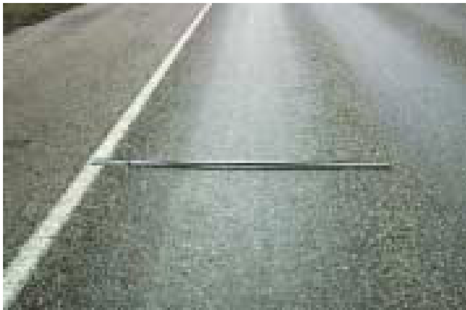
Figure 4.2.1 Road Pavement Rutting
