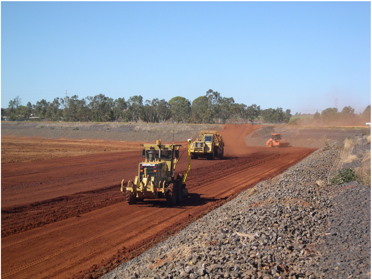
Figure 9 Trimble Precision GPS Real Time Machine Guidance Trial, Dubbo City Council Effluent Ponds Reconstruction, May 2007
