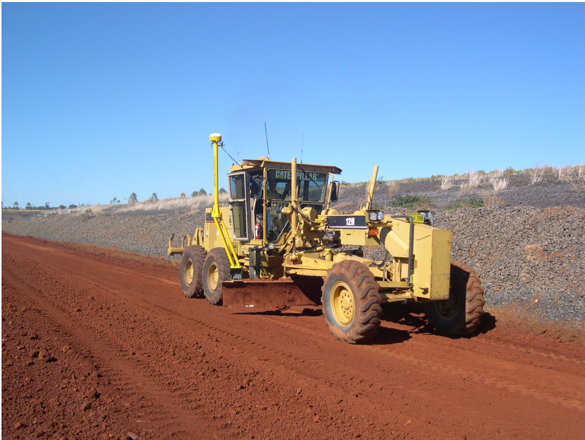
Figure 8 Trimble Precision Guidance infrastructure fitted to DCC grader - GPS Real Time Machine Guidance Trial, Dubbo City Council Effluent Ponds Reconstruction, May 2007
