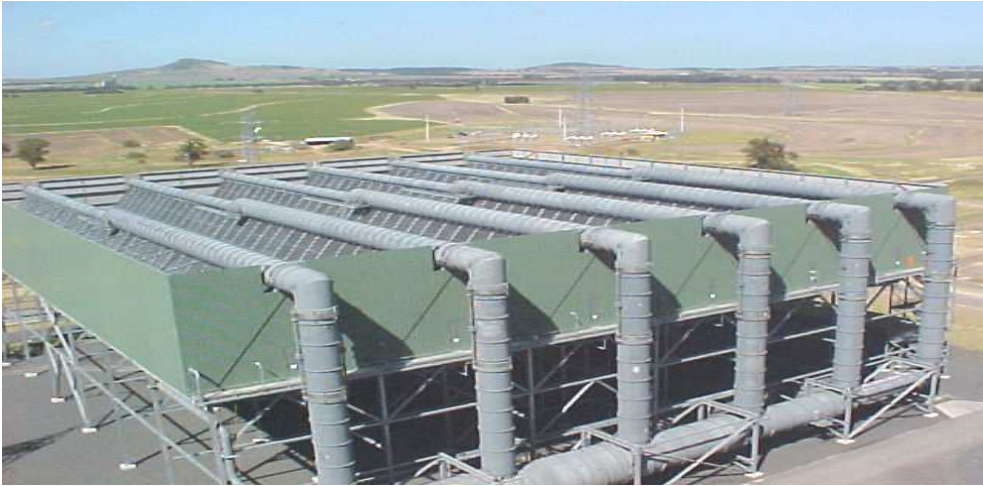
Figure 2-4 Millmerran power plant air-cooled condensers
