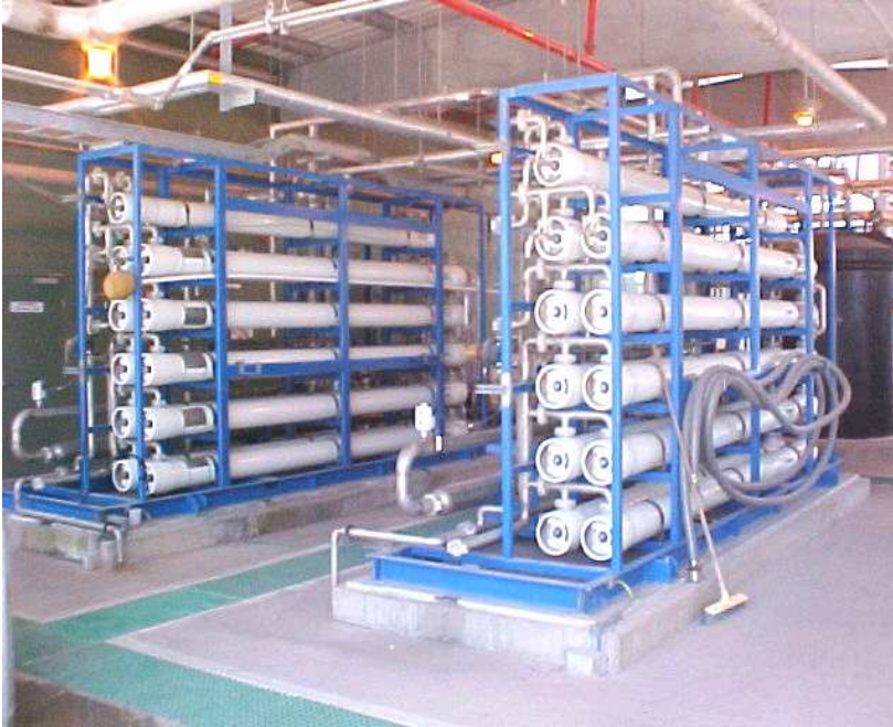
Figure 2-10 Millmerran power plant reverse osmosis water treatment unit
