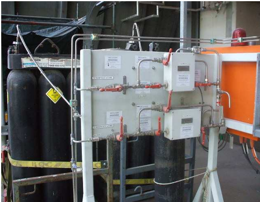
Figure 4-10 Oxygenated treatment control valve panel
