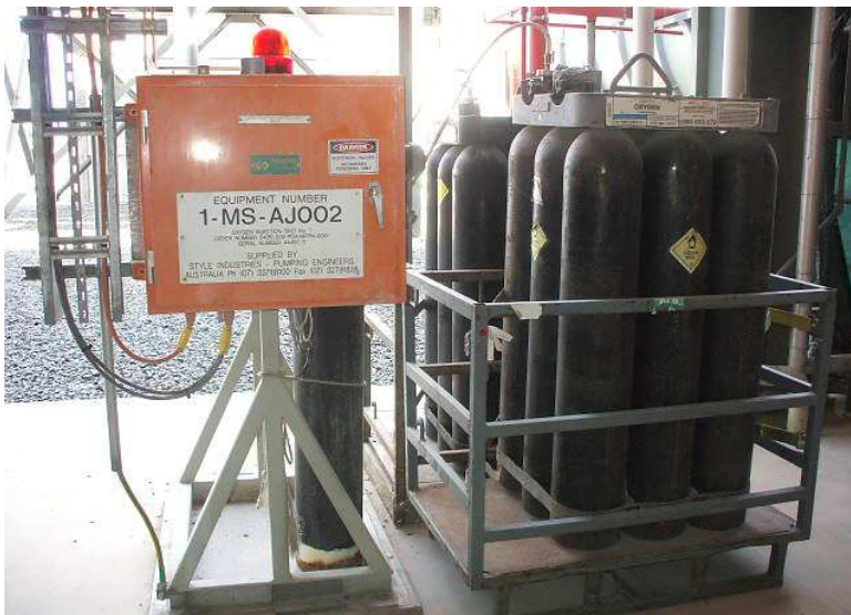
Figure 4-3 Oxygenated Treatment Skid
