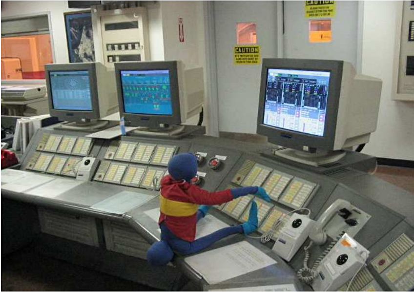
Figure 3-8 Millmerran power plant control room (DCS) configuration
